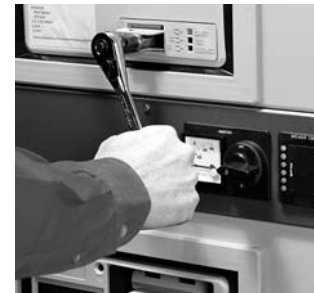
Drawout Breaker Levering Can be Accomplished With the Compartment Door Closed Without the Need for a Special Levering Tool
